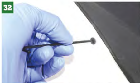
You'll need to enlarge the Cleco hole in the arch to provide clearance for the fixing screw. These are M4x16 mm countersunk head Allen screws, which Matt will also fit screw cups to, making the installation neater — although he may increase the screws' lengths to 20 mm.
