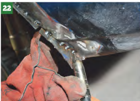
22 ...all you now have to do is tack it to the outer skin and work your way round — as usual, do small sections at a time and keep checking you're not distorting the arch.
