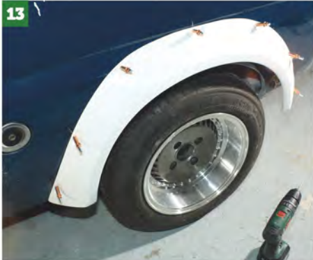
13 Once completely fitted stand back and check it's all as you want it and that the wheels fit the arch.
