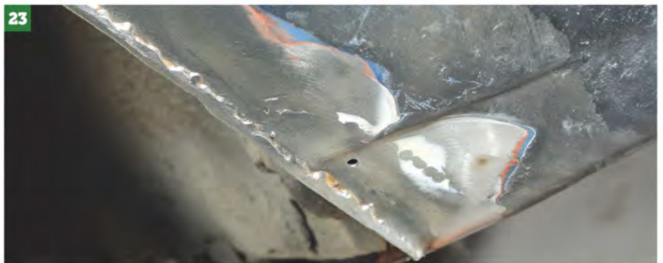
23 When you're happy with the tacks, you can finish weld them shut — but again, do small sections at a time to control heat and subsequent distortion.
